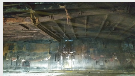
Image 2: The garage deck No.3 following the fire
